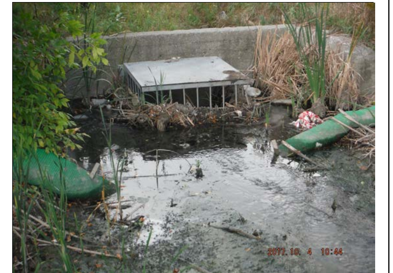
Photo 40: Downstream vertical culvert acting as a permanent barrier to fish passage upstream
