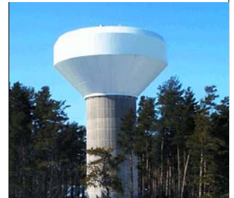
Current groundwater supplies will not meet the projected growth and demand in Newmarket and Aurora.
