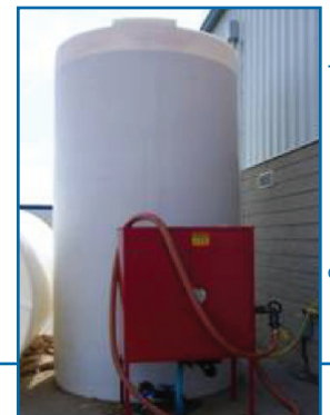
Liquid Salt Brine Storage Tower
