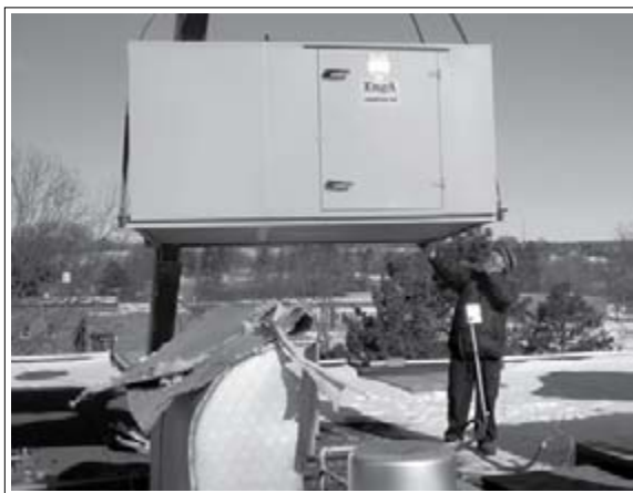
A new make-up air system being placed on the roof by crane at Pineview Terrace in Keswick.
