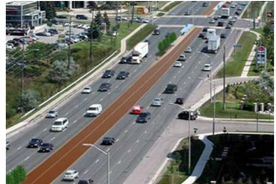
Viva Phase 2 involves constructing centre-of-the-road lanes known as "rapidways", dedicated strictly to public transit.
