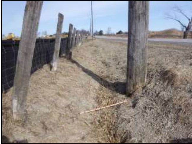
Photograph 17. (Location 6) Bruce Creek Tributary Reach BR2-H15 North facing view of ROW along western side of Warden Avenue at BR2-H15.
