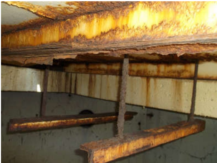
Figure 2-11. Condition of Interior Roof of South Elevated Tank
