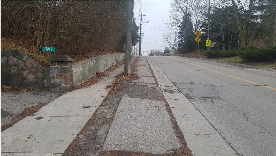
Image 1: View of disturbances associated with the asphalt roadway, concrete shoulder, curbs and sidewalk, and cut slope with concrete barrier.
