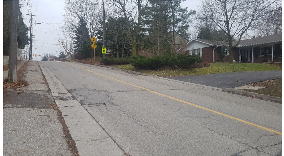
Image 2: View of disturbances associated with the asphalt roadway, concrete shoulder and curbs, intersecting driveways and residential structures.
