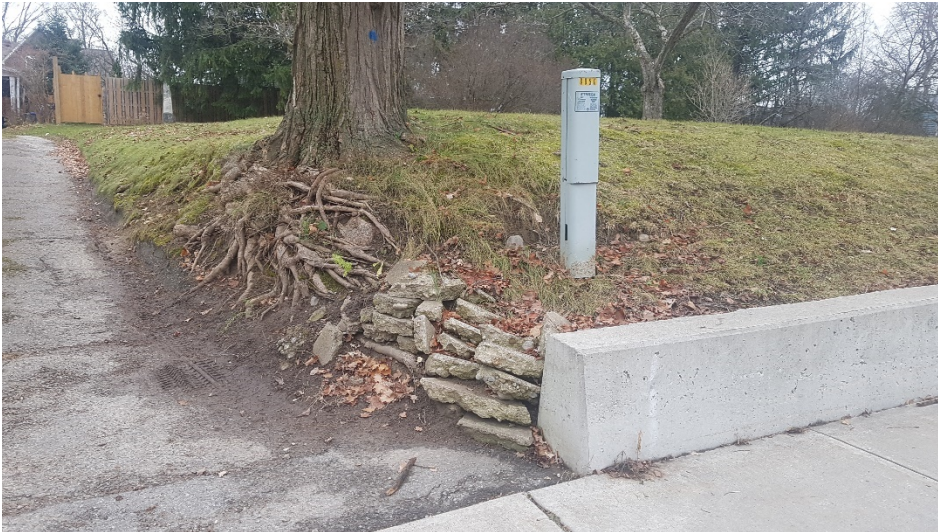
Image 5: View of disturbances associated with a cut slope, concrete barrier, sidewalk, driveway and utilities adjacent to the Mount Albert Wesleyan Methodist Pioneer Cemetery limits.
