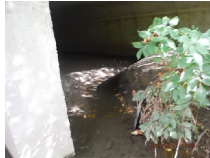
Photo 31: Downstream woody barrier
