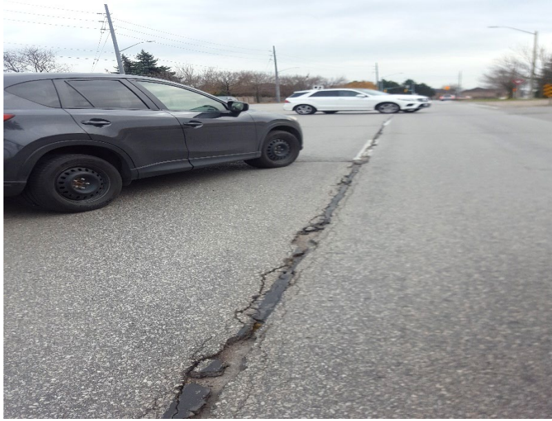
Photo 7 – Severe longitudinal joint cracking between southbound lanes 1 and 2, north of Carlton Road.
