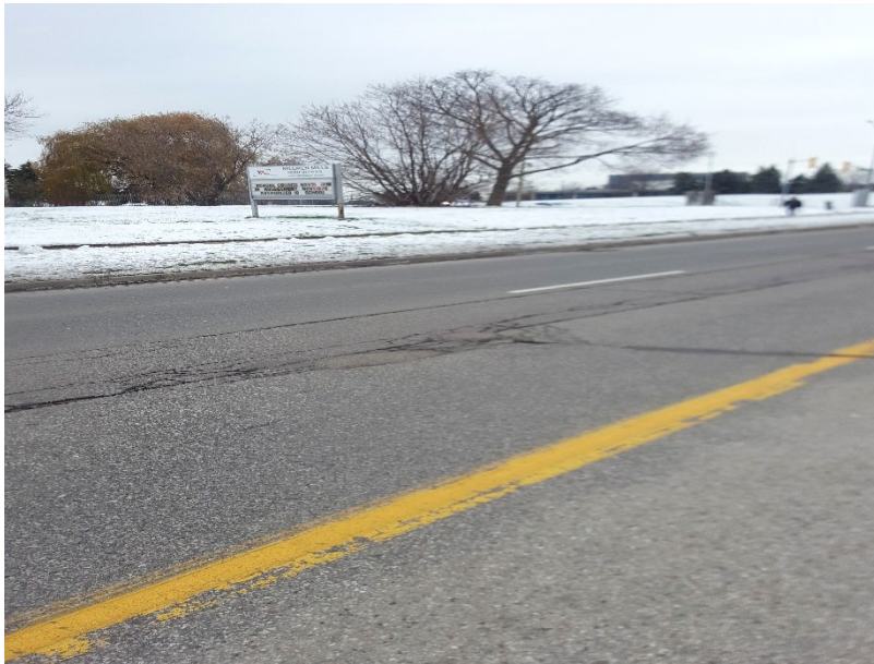
Photo 8 – Severe longitudinal and transverse cracking in southbound lane 1, south of Highglen Avenue.
