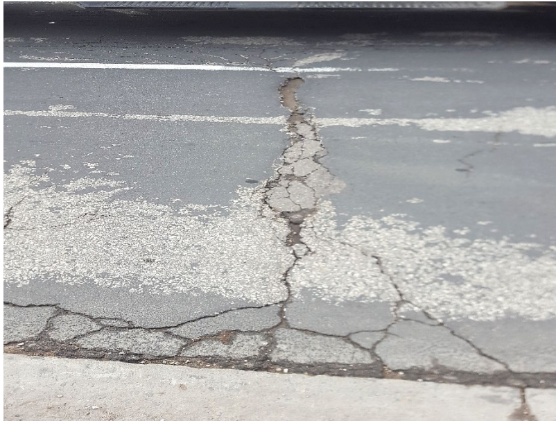
Photo 16 – Severe transverse alligator cracking in northbound right-turning-lane, south of Highway 7.
