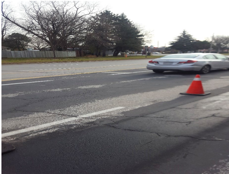
Photo 6 – Moderate severity transverse and longitudinal cracking in southbound lane 2, north of Highway 7.
