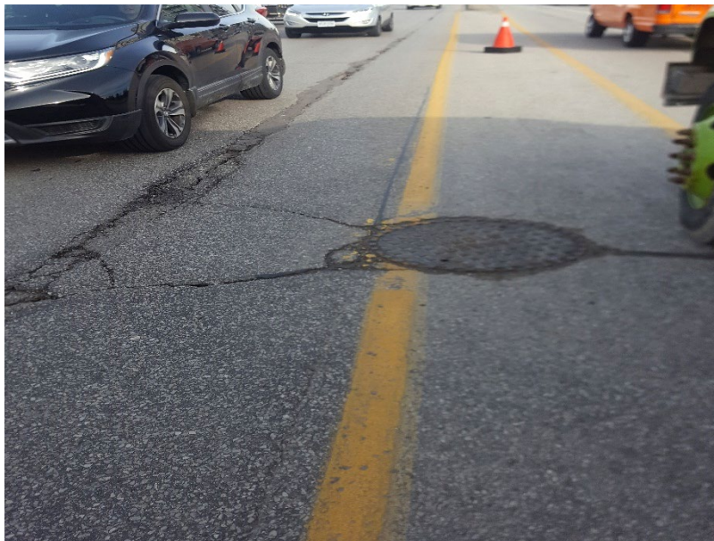
Photo 12 – Severe longitudinal cracking along northbound lane 1, north of Helen Avenue.
