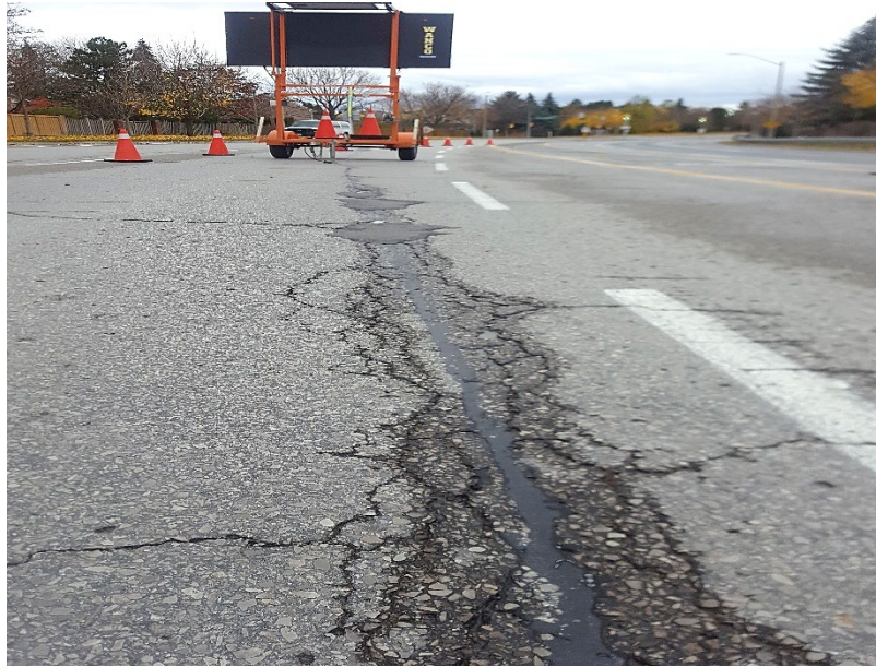
Photo 1 – Severe longitudinal alligator cracking in southbound lane 1, south of 16 th Avenue.
