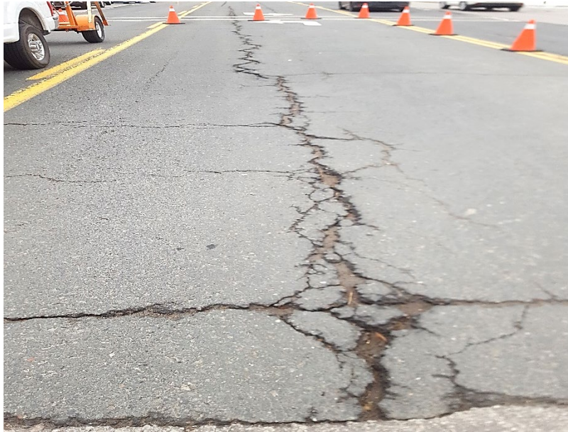
Photo 11 – Severe longitudinal and transverse cracking in the shared left-turning-lane, south of 14 th Avenue.
