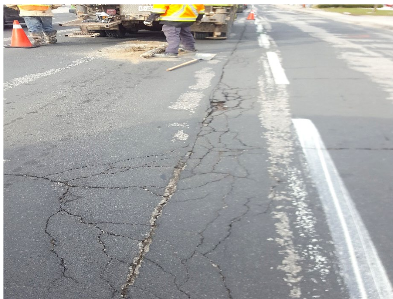
Photo 14 – Moderate severity longitudinal and alligator cracking along northbound lane 2, south of Highway 7.
