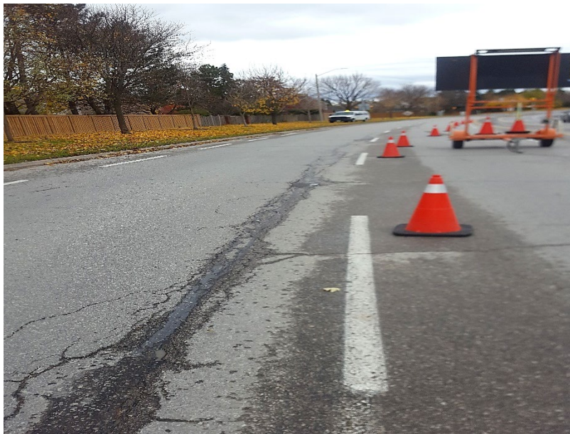
Photo 2 – Severe longitudinal cracking in southbound lane 2, south of 16 th Avenue.
