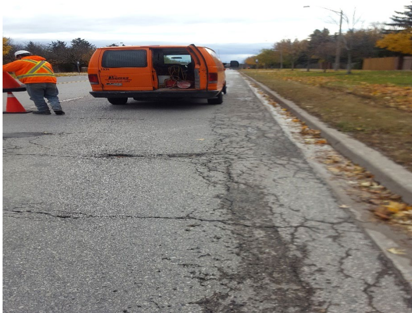
Photo 4 – Severe alligator cracking in the right wheel path and transverse cracking in southbound lane 2, north of Carlton Road.
