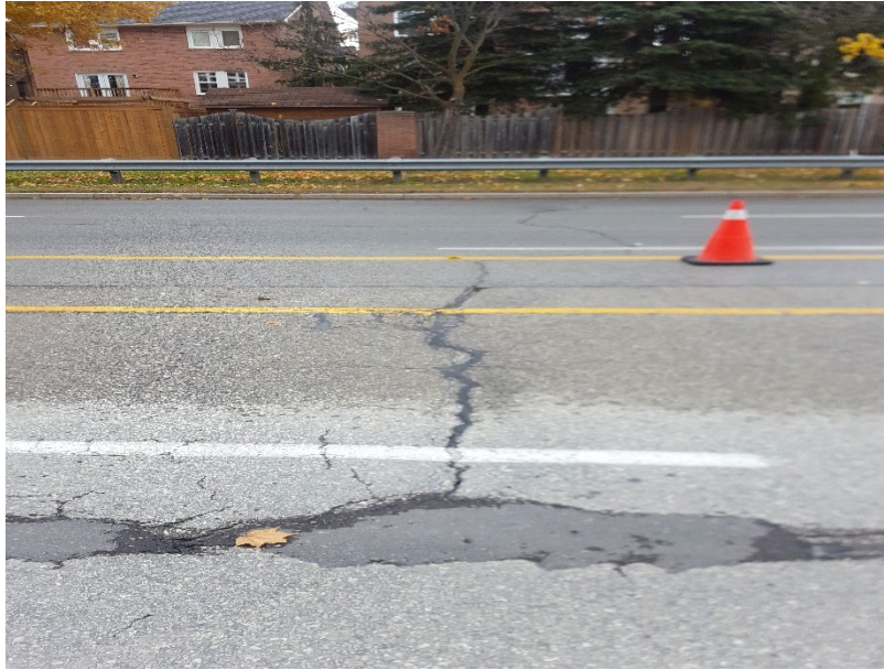
Photo 3 – Severe transverse cracking across all lanes and machine patched pothole in southbound lane 2, south of 16 th Avenue.
