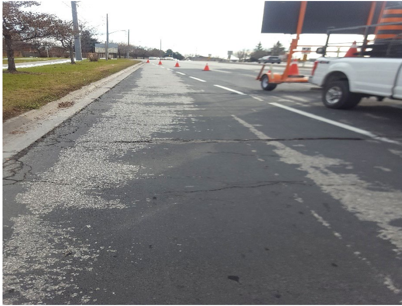
Photo 15 – Severe transverse cracking and raveling in northbound right-turning-lane, south of Highway 7.
