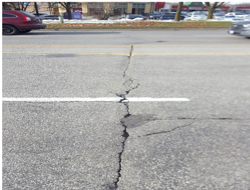
Photo 13 – Severe transverse cracking across northbound lanes 1 and 2, north of Castan Avenue.
