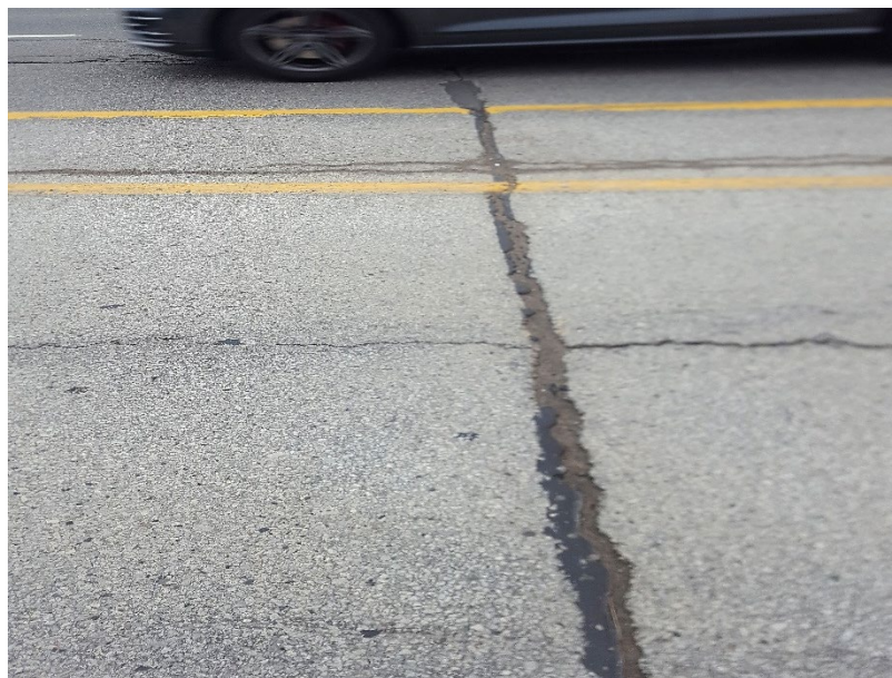
Photo 10 – Severe transverse cracking in northbound lane 1, south of Highglen Avenue.
