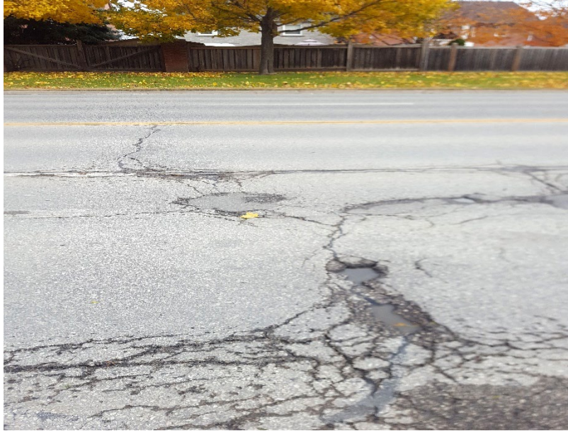
Photo 5 – Severe alligator and longitudinal joint cracking and potholes in southbound lane 2, north of Carlton Road.
