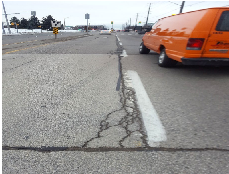
Photo 9 – Severe longitudinal joint cracking between lanes 1 and the left-turning-lane, south of Highglen Avenue.
