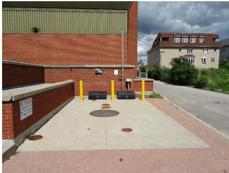
Photo 3 – UST with overfill alarm at Bell, 7733 Kennedy Road (Section 1, facing east)
