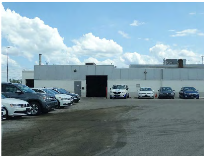
Photo 5 – Hydrocarbon staining on concrete at Volkswagen Dealership and Service Centre at 7997 Kennedy Rd (Section 2, facing south)
