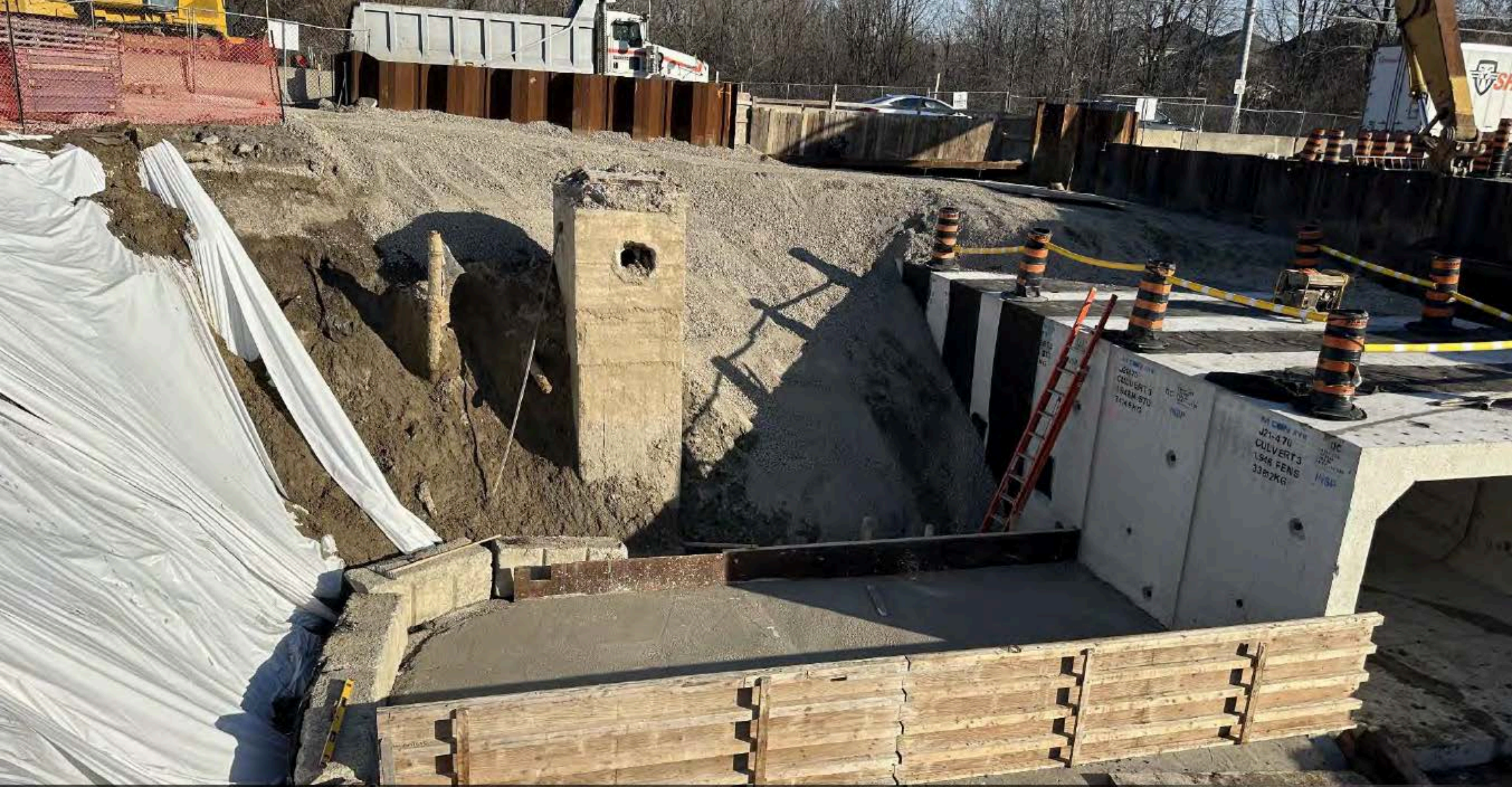
Concrete footing for south wingwall on Rutherford Road, west of Greenock Drive
