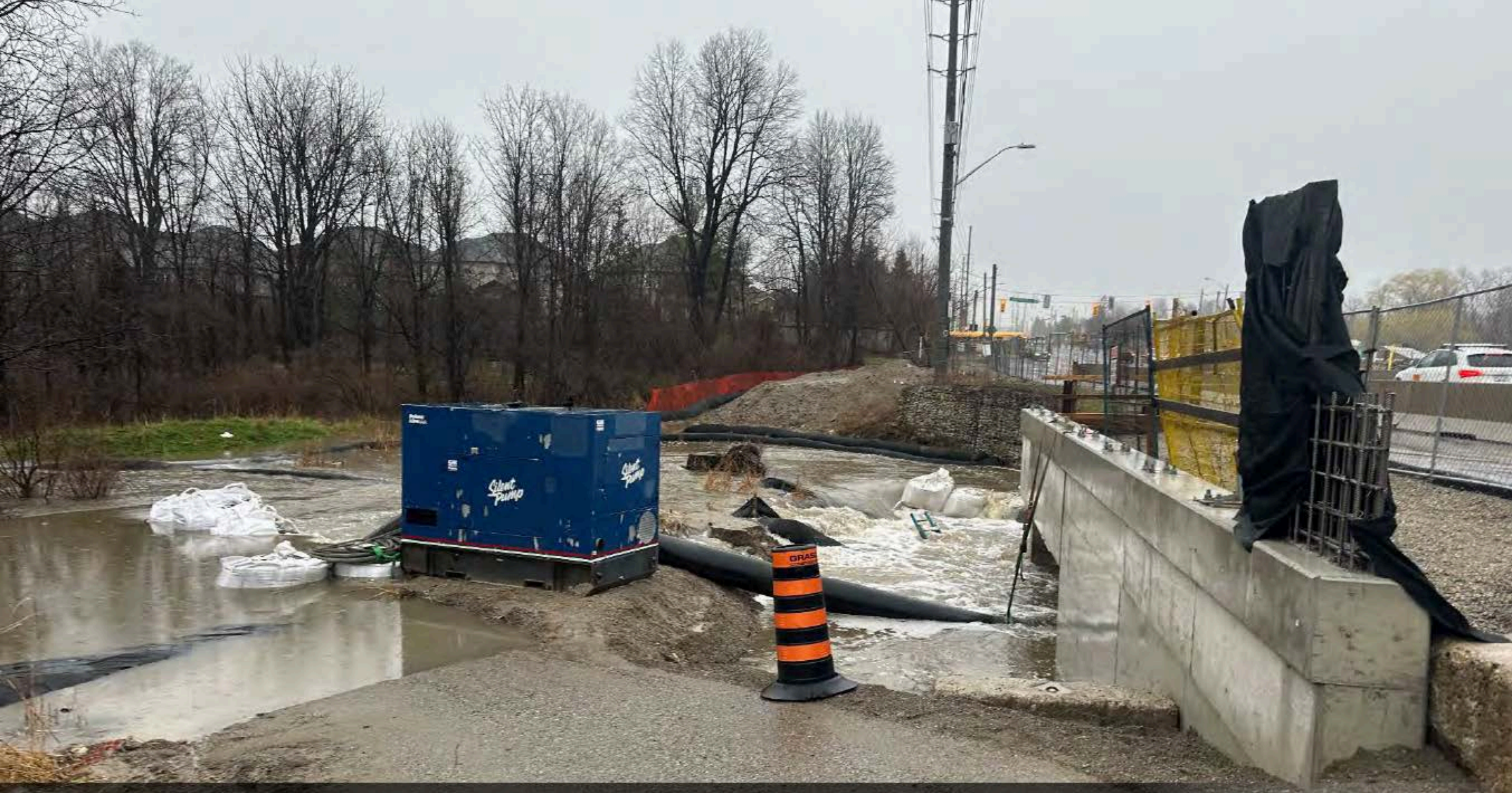
Work at culvert paused due to high water levels on Rutherford Road, west of Greenock Drive
