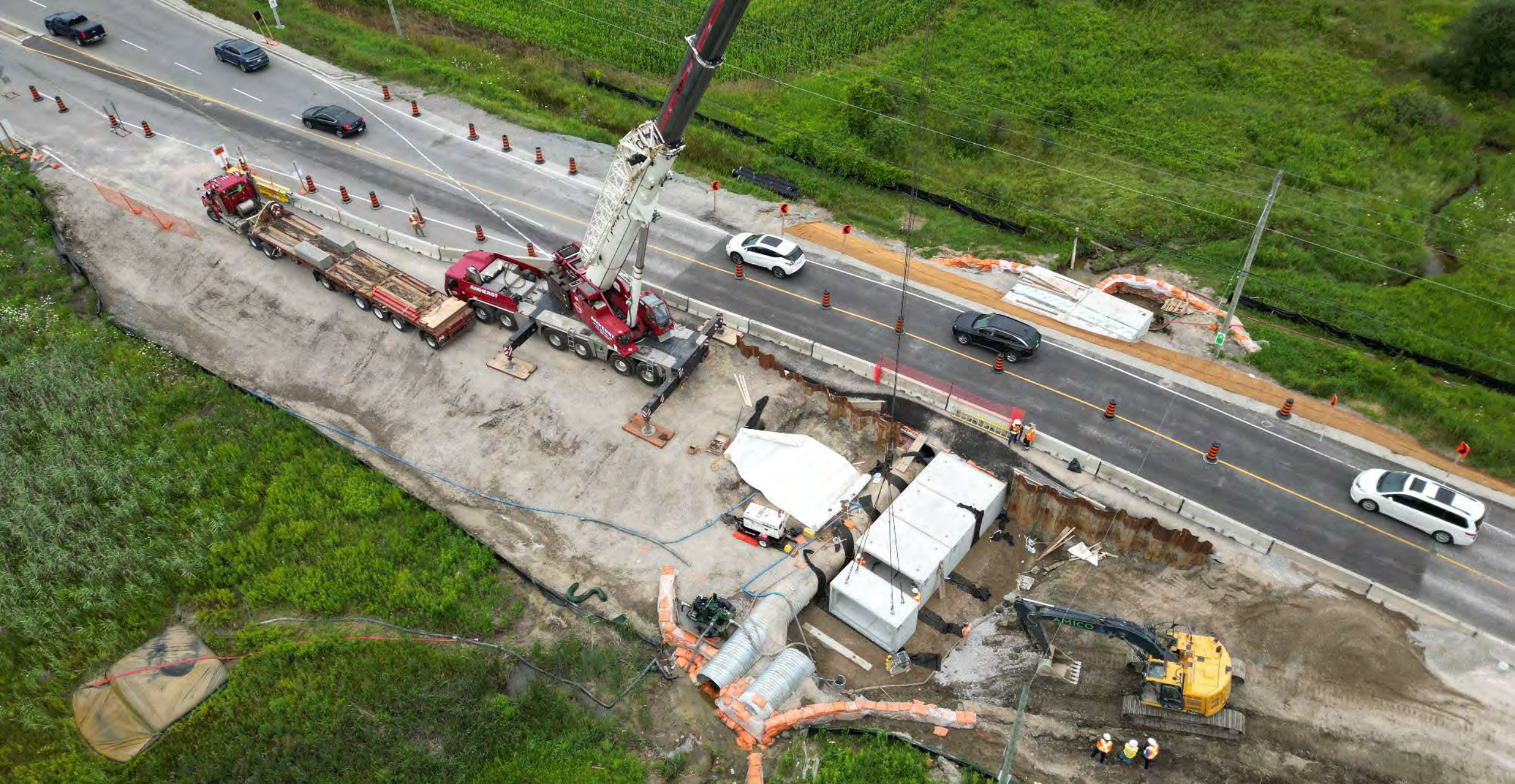
New larger culvert being installed on Rutherford Road, east of Jane Street
