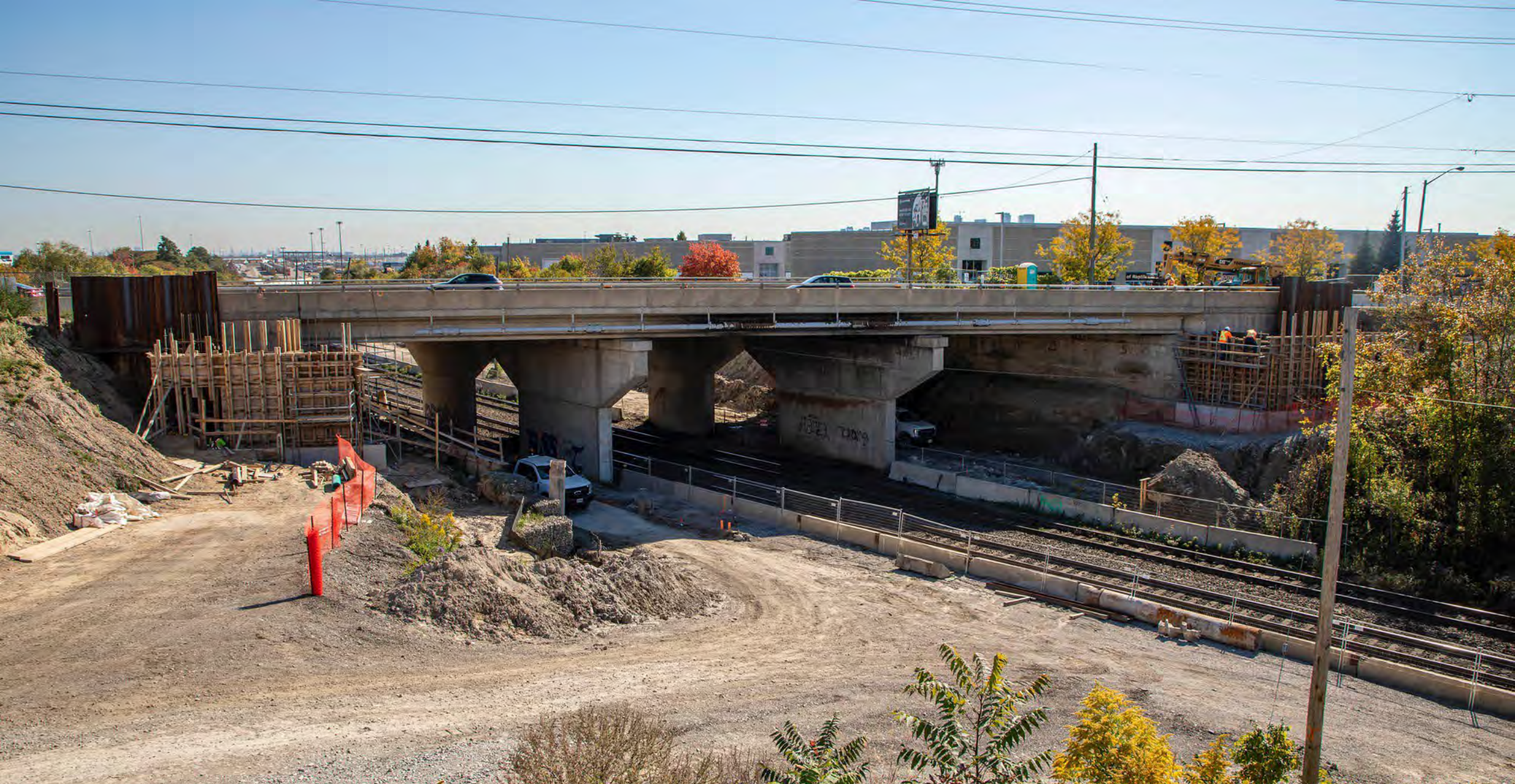
Access road and construction of bridge abutments to widen bridge over CN Rail tracks
