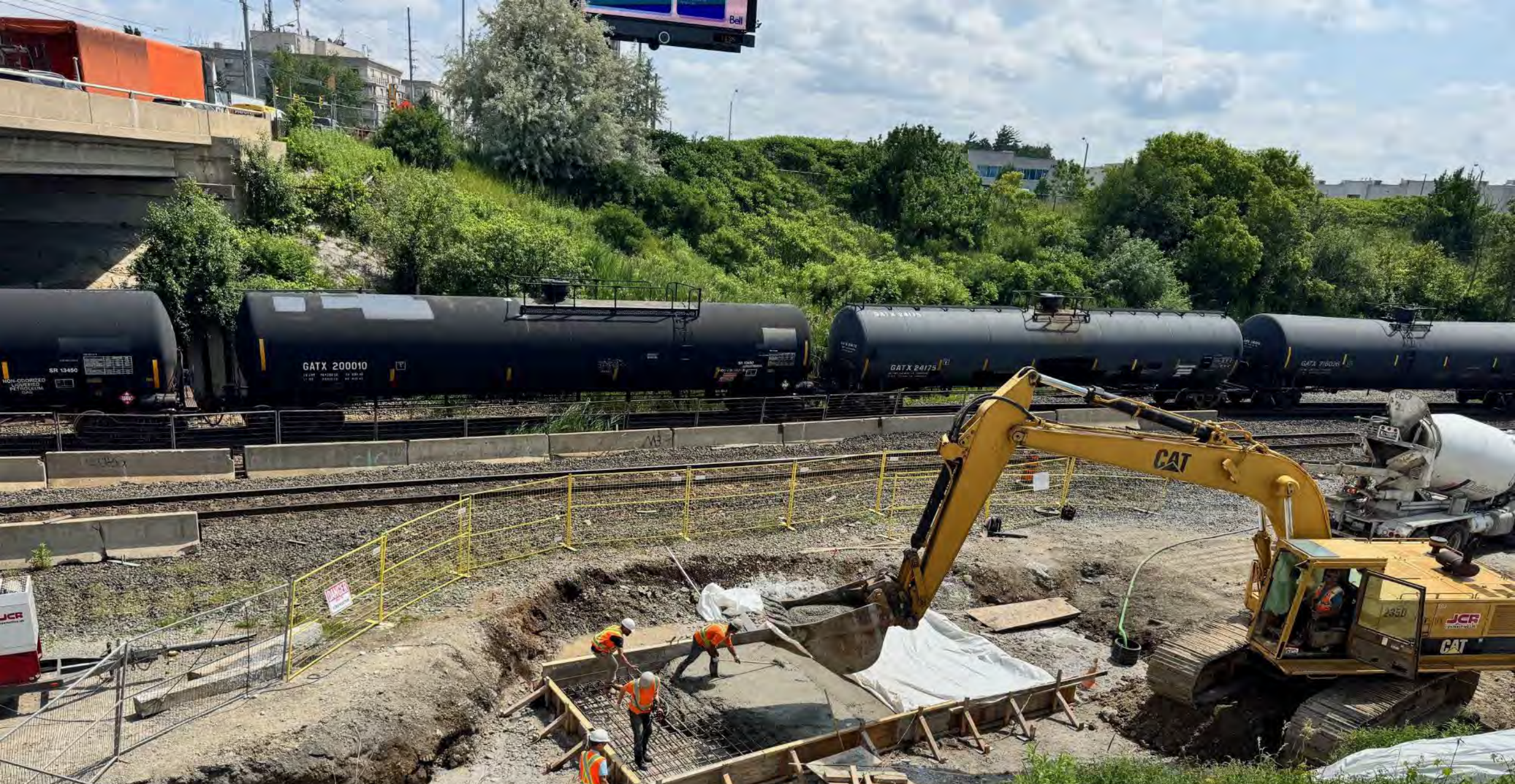
Watermain protection installation under CN Rail bridge on Rutherford Road, City of Vaughan
