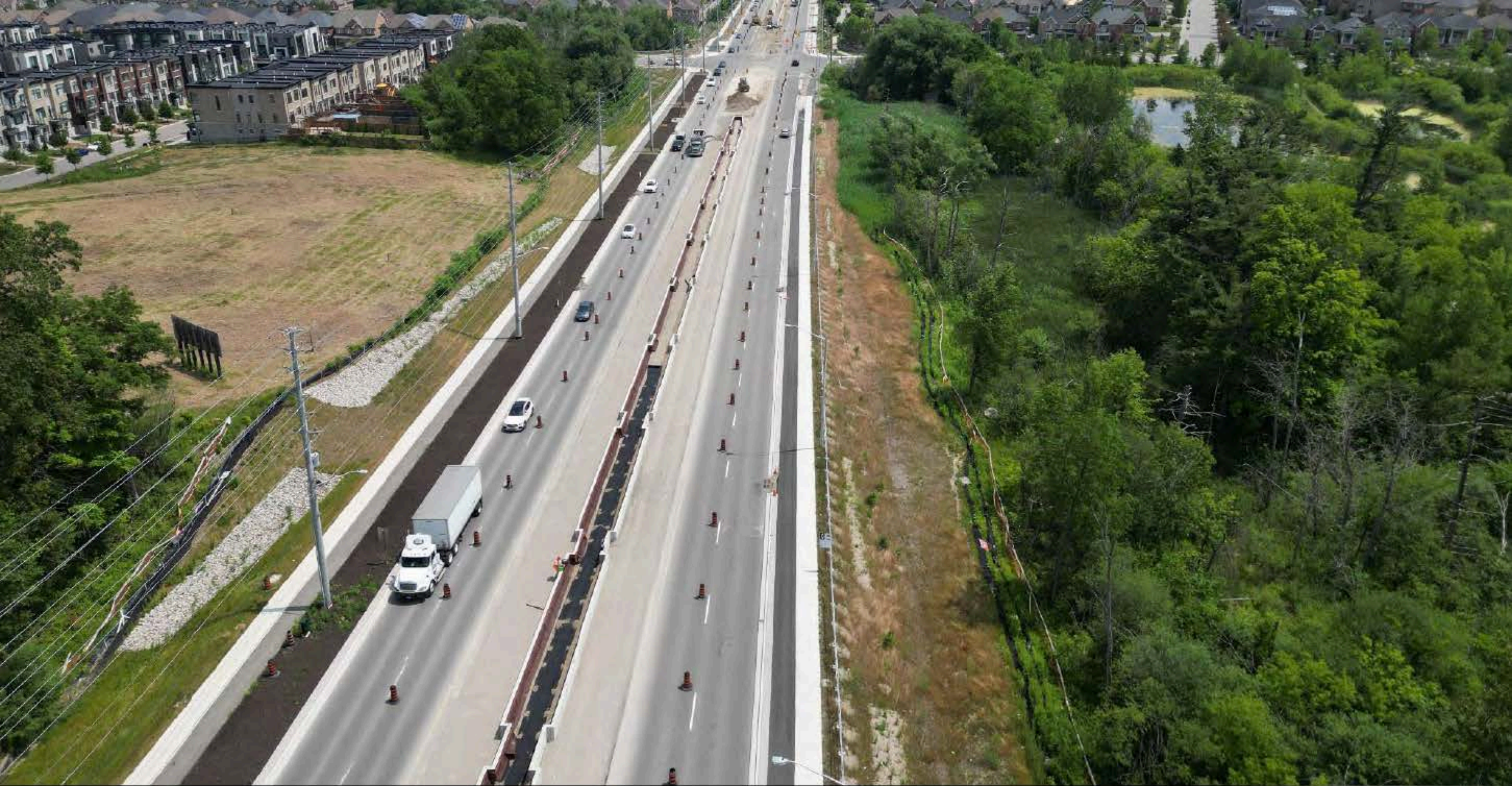
Road widening and median construction on Rutherford Road, looking east from Dufferin Street
