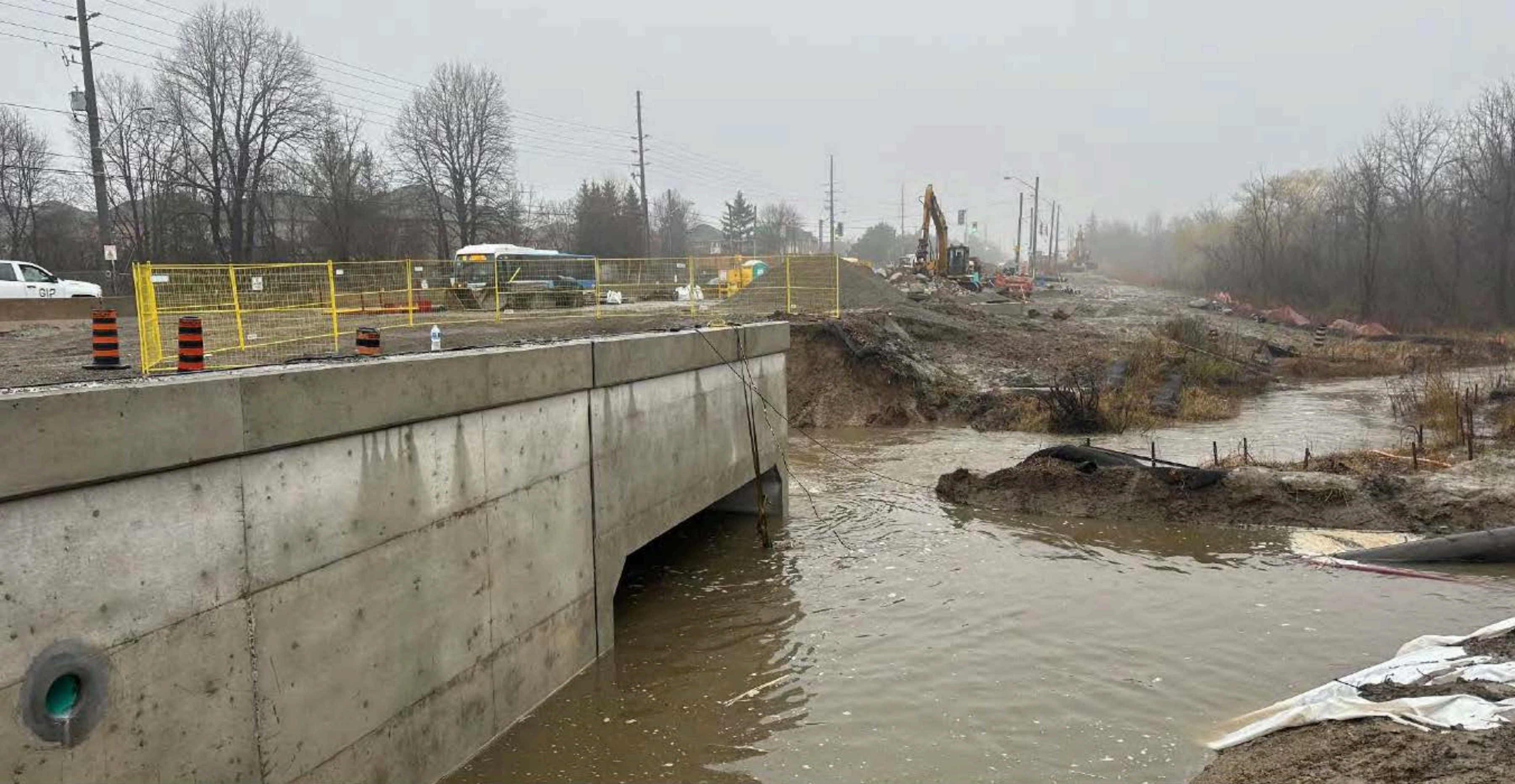
Work at culvert paused due to high water levels on Rutherford Road, west of Greenock Drive
