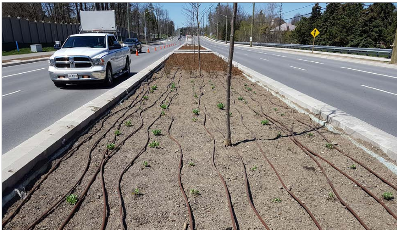
A landscaped center median with dripline irrigation laid out before plant material is installed.
