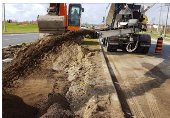
A soil slinger installing the Engineered Growing Media in a median soil trench.
