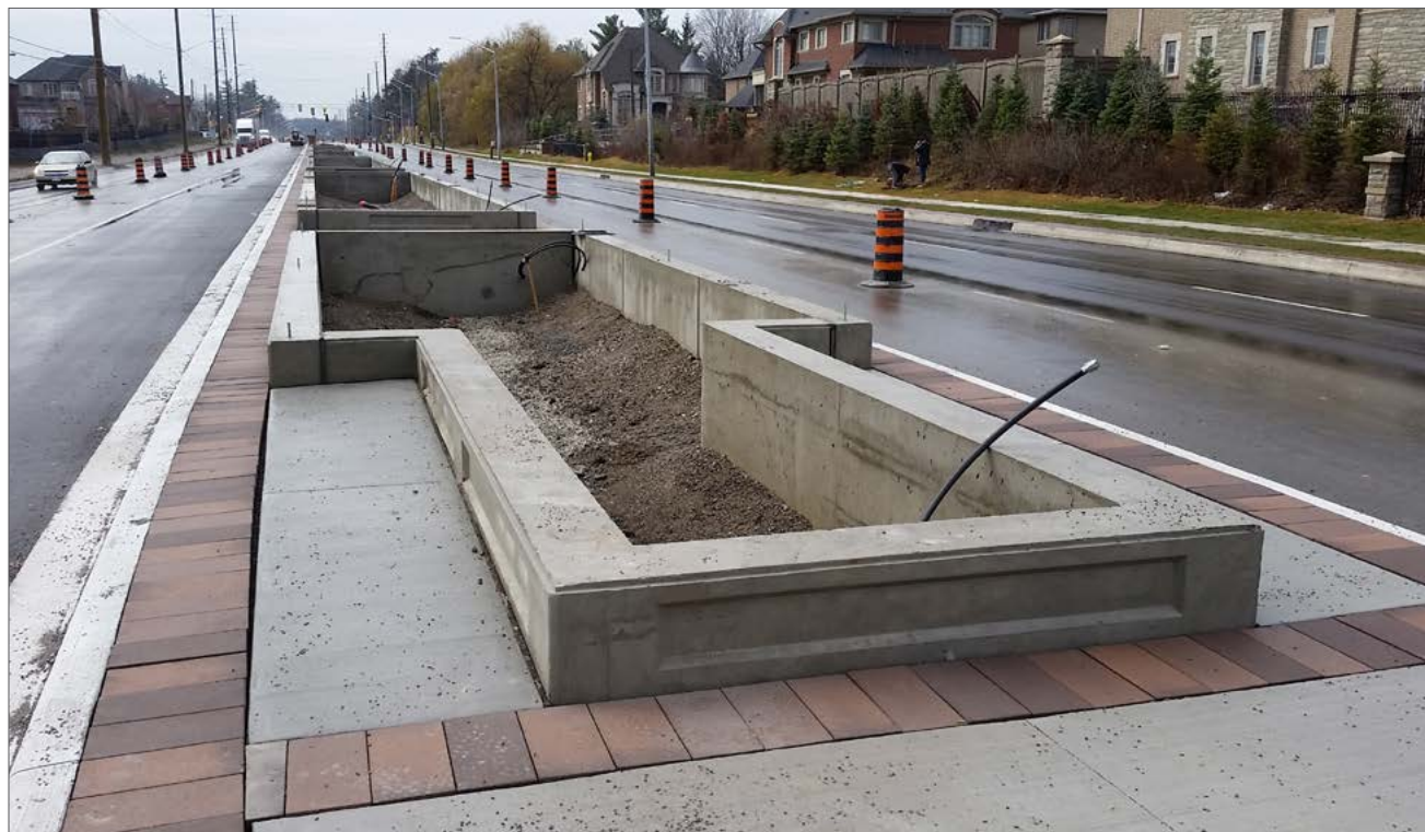
A landscaped center median planter before the Engineered Growing Media, trees and plant materials are installed.
