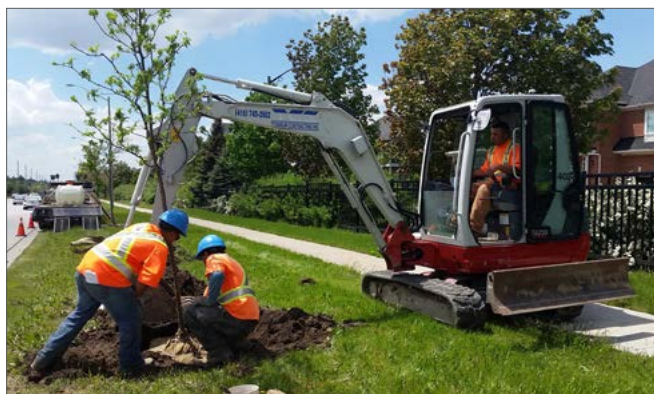
Tree planting contractor utilizing a mini excavator for proper tree placement in the boulevard.
