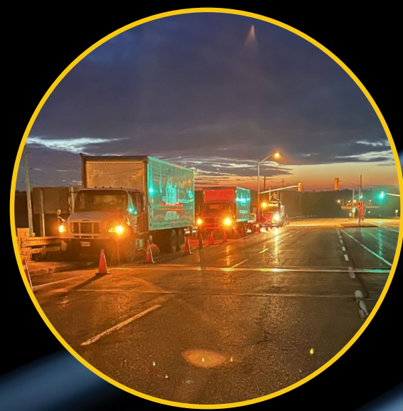
YorkNet crews constructing highway crossing at Highway 404 and Queensville Sideroad in the Town of East Gwillimbury
